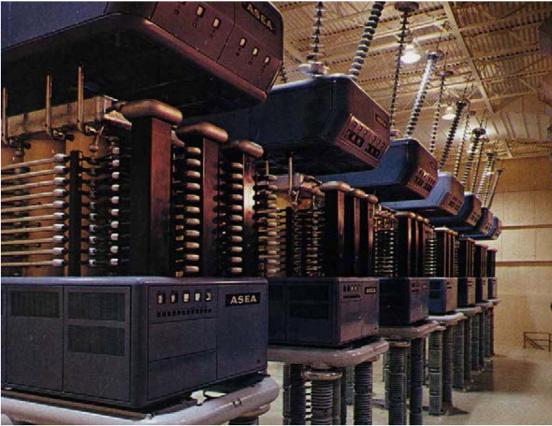
Mercury-arc valves Pacific Intertie Photo: Hitachi Energy
