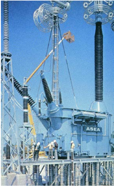
Transformer for ultra-high voltage (UHV) at the AEP-ASEA Test Station in South Bend, Indiana USA. Foto: Hitachi Energy
