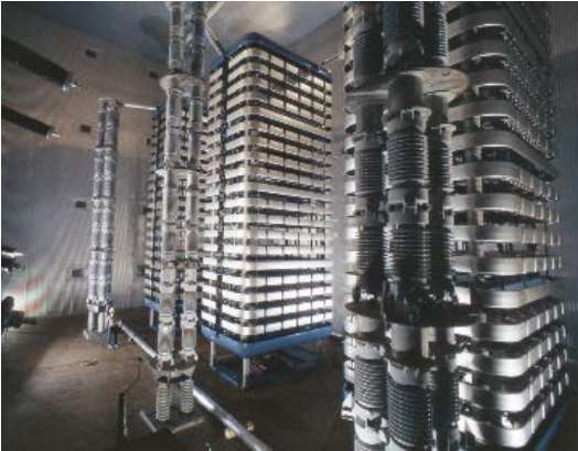
Water-cooled standing valves in 300 kV hall for Itaipu Photo: ASEA, Västmanlands läns museum
