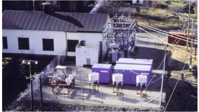
Hellsjön Converter Station adjacent to Hellsjön Hydropower Station Photo: Hitachi Energy
