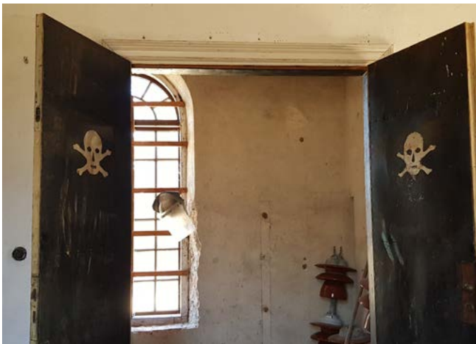
Even today, original interiors remain in Hellsjön's Power Station - here the doors to the switchgear room. Photo: Tommy Hjort
