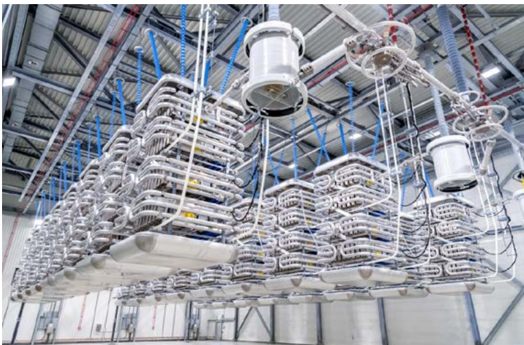
Water-cooled suspended IGBT valves for NordLink Photo: Hitachi Energy
