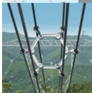
AEP 765 kV Interstate project
