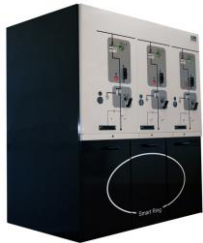
MV breaker cubicles
